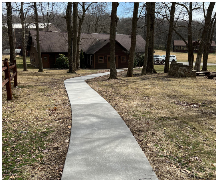
The path leading up to the "Mon" with a concrete rebuild for better accessibility
